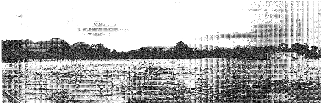
Figure 1: Picture of EAR installed at Koto Tabang, West Sumatra, Indonesia
