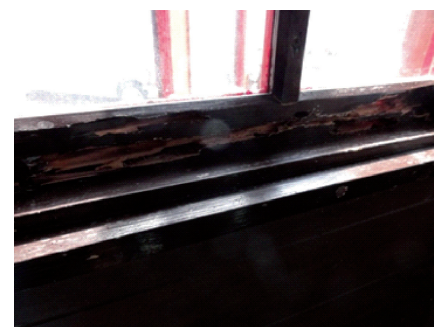
Fig. 1. Window sill infested with drywood termites, Nobeoka, Kyushu, March 12, 2011
