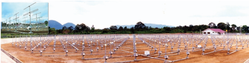
EAR antenna field (110 m diameter, 560 Yagi antennas, 100 kW peak output power)
