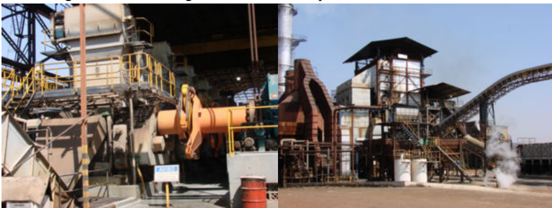
Fig. 6 Left: steam turbine driven mills. Right: boiler.
